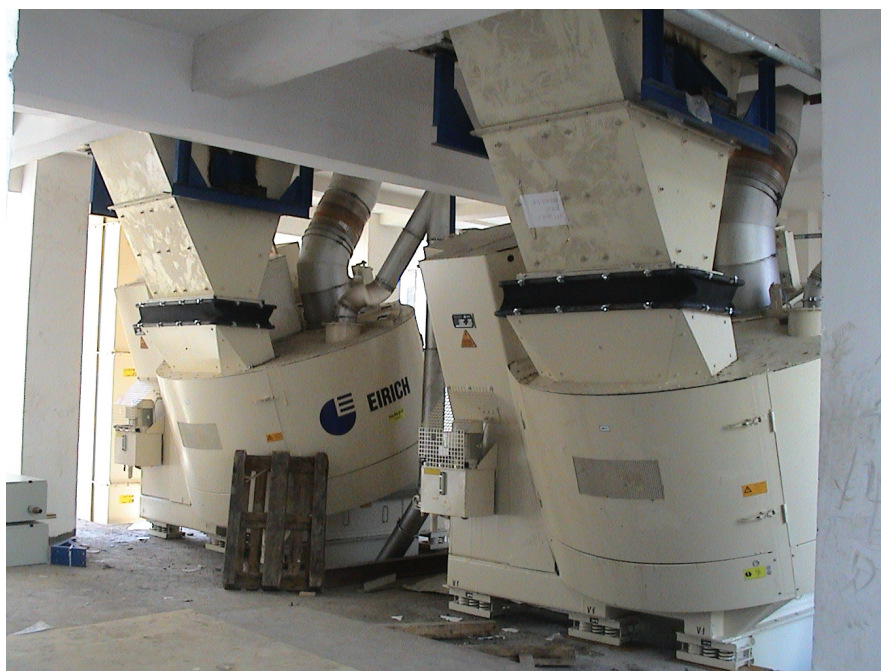
This photo was taken immediately after the installation of two Type R 24 intensive mixers at a Philips glass-making plant in China. Philips began manufacturing in China in 1984, and the company is now firmly established in the electronics market there.
