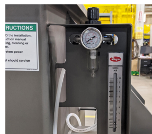
Shaft seal filter regulator gauge
