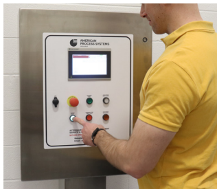
Paneles de control
