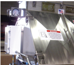
NEMA 4/12 water tight timer and Magnehelic differential pressure gauge
